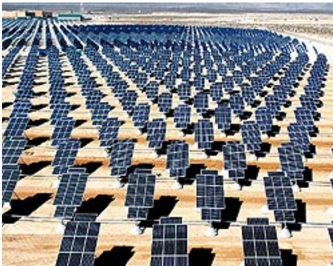
Figure 2. Single axis tracking photovoltaic array, Nellis Air Force Base, Nevada
